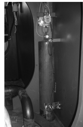
Figure 1. Measurement of piston rod position using an encoder in a press machine
