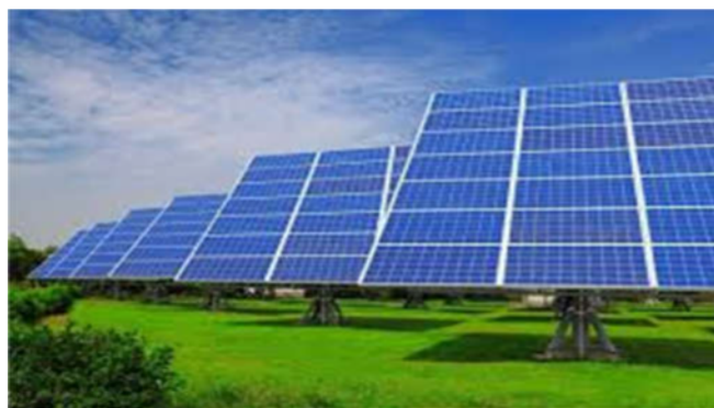
Figure 3. Solar power plant
