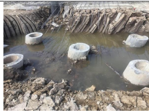
Figure 6. Pile movement at axis A during Excavation and construction of pile cap
