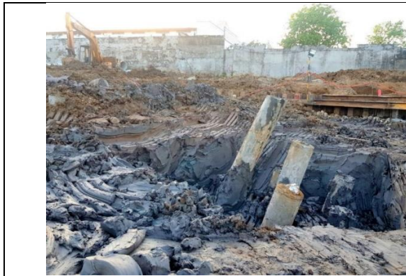
Figure 5. Pile movement at axis A during Excavation
